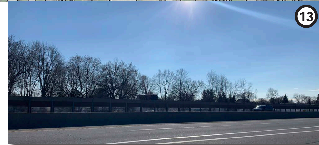
Noise barrier wall along the southern edge of Highway 401 screens view into the adjacent residential areas. Some vegetative buffer is provided between the highway and noise barrier.
